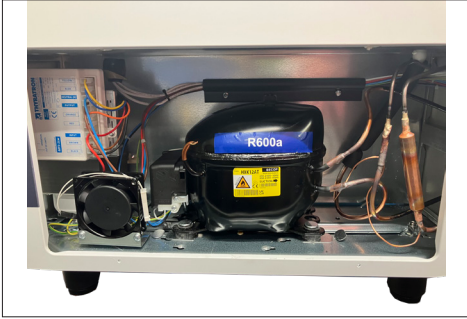
1. The Voltage stabilizer is placed on the left side of the compressor compartment
