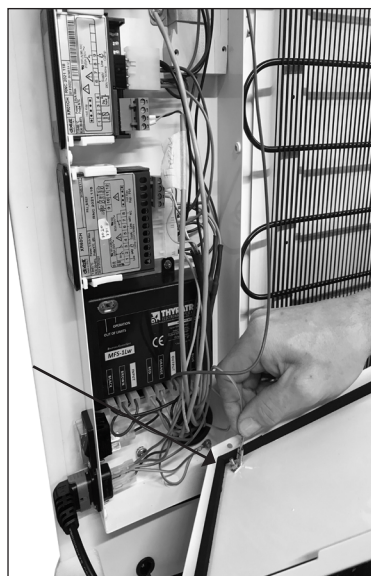
2. Remove grounding cable from junction box by unscrewing bolt with a wrench 6mm.
