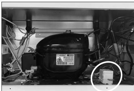
1. Valve to be replaced
