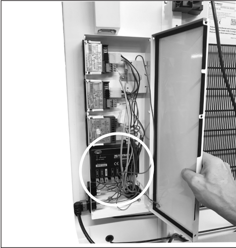
1.The controller is placed in the bottom
