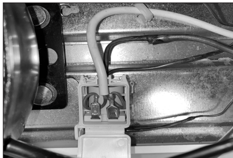
2. Valve to be replaced
