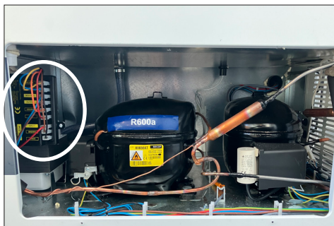
1. The transformer is placed on the left side of the compressor compartment behind the Voltage stabilizer
